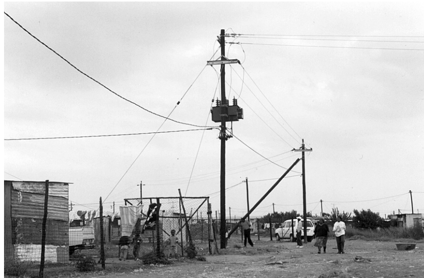
Figure 2: Bare MV and abc LV overhead conductors
