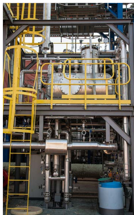
Bokpoort concentrated solar power plant near Groblershoop
