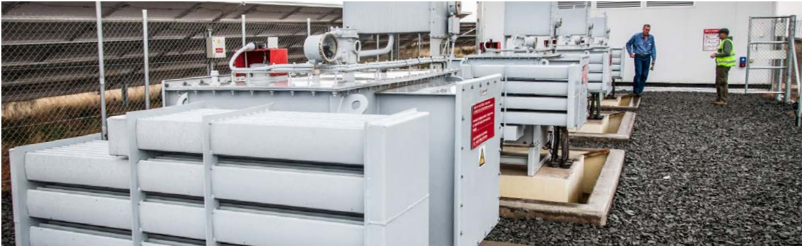
De Aar Solar Power PV plant near De Aar
