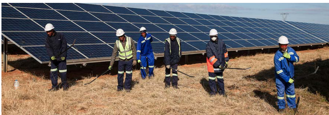
Droogfontein solar power PV plant near Kimberley
