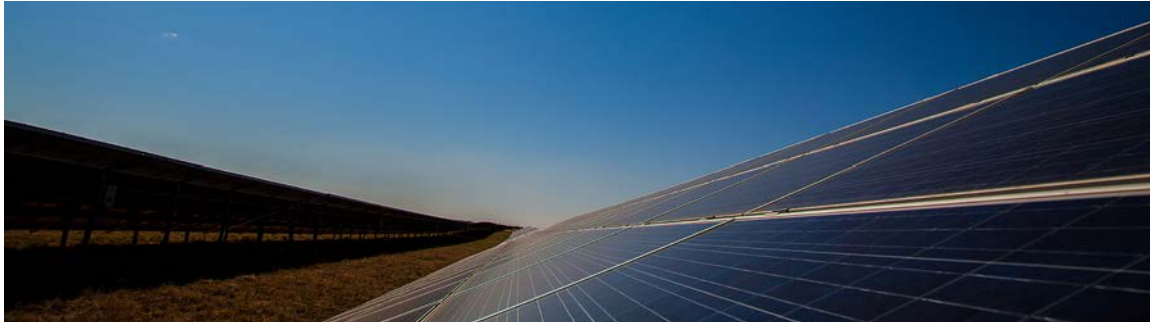
Droogfontein solar power PV plant near Kimberley
