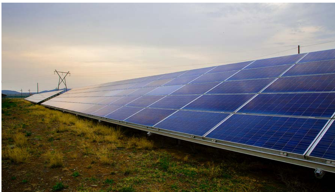
De Aar Solar Power PV plant near De Aar
