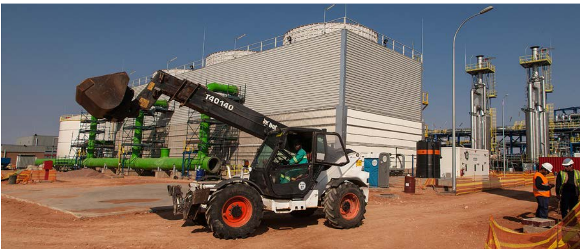
Bokpoort concentrated solar power plant near Groblershoop
