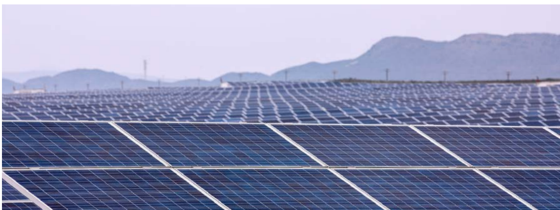
De Aar Solar Power PV plant near De Aar
