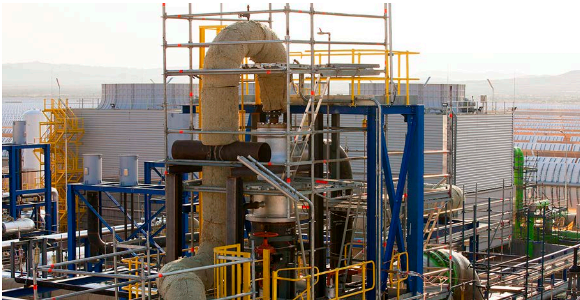
Bokpoort concentrated solar power plant near Groblershoop
