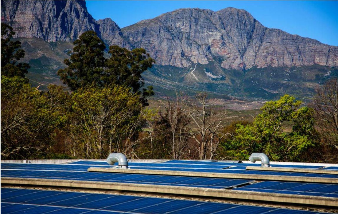
Sustainable Power Solutions Rooftop PV installation at Lourensford Wine Estate near Somerset West
