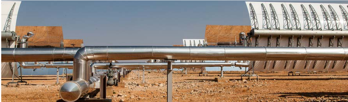
Bokpoort concentrated solar power plant near Groblershoop
