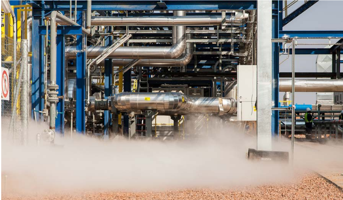
Bokpoort concentrated solar power plant near Groblershoop
