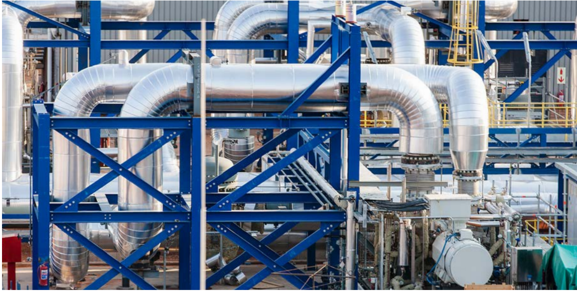
Bokpoort concentrated solar power plant near Groblershoop
