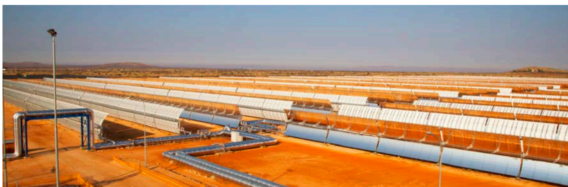
Bokpoort concentrated solar power plant near Groblershoop
