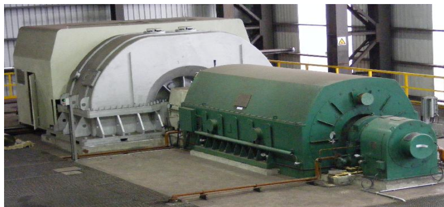
Fig. A.4-6: The general view of the steam turbine and alternator
