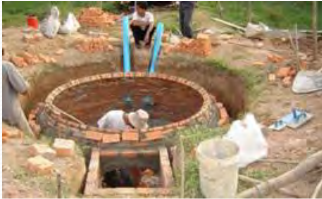
Constructed fixed dome-Giyani Project
