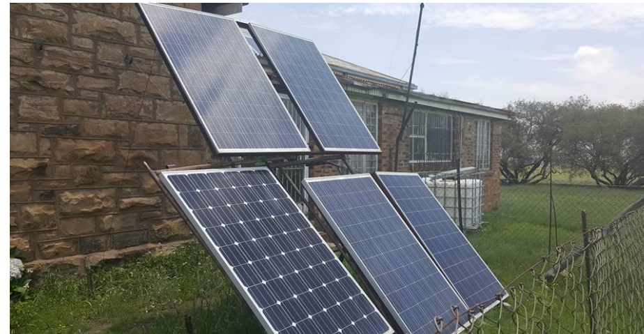
Solar PV village electrification
