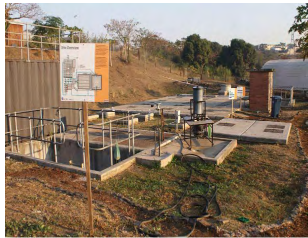
Dewats Plant – EThekweni
