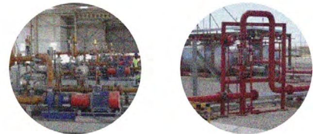
Steam Turbine Enclosures
