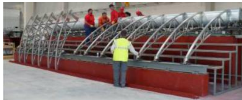
Collector structure - Spain
